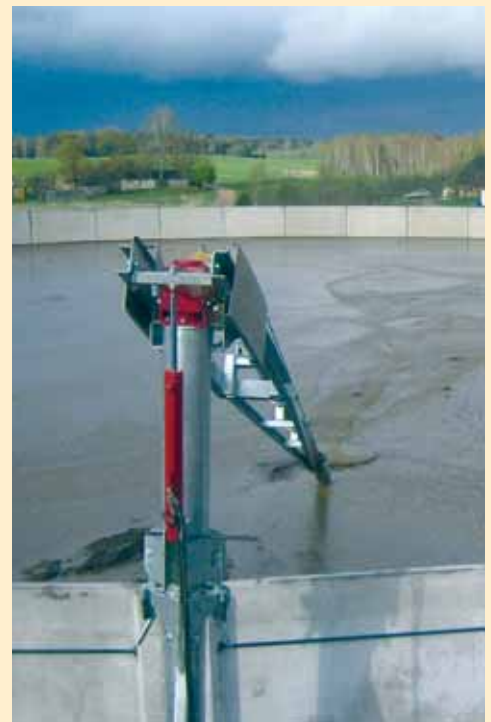
Complete homogenisation of the settlings and floating crusts
